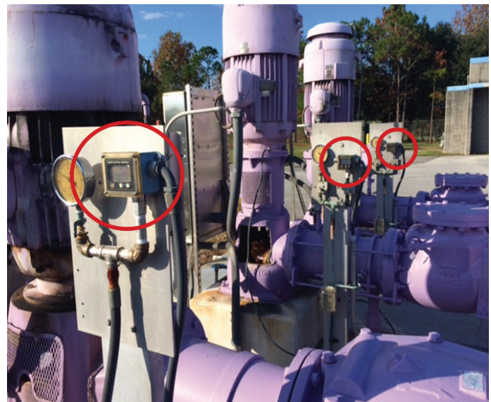
Electronic switch mounted on pump systems in a water facility
