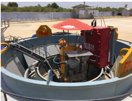
Rim Seal Fire Protection System on top of a storage tank
