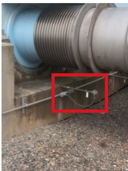
Figure 2. Temperature sensor to detect LNG leaks at the base of an LNG storage tank.
