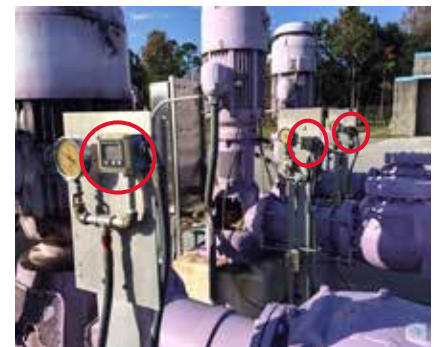
IMAGE 2: Electronic switch mounted on pump systems in a water facility
