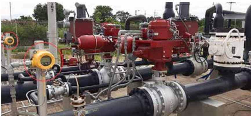
IMAGE 2: Pressure switch installed on pump system
